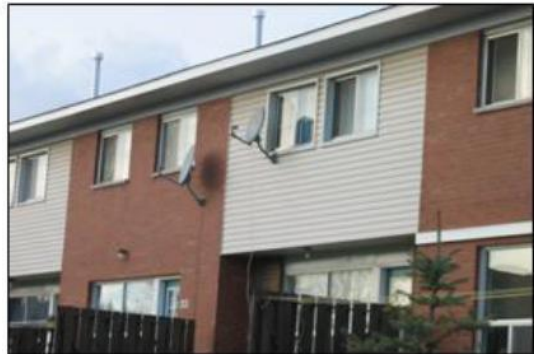
Fastened to Siding
