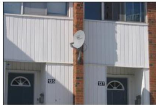
Fastened to Brick Wall Outside Unit
