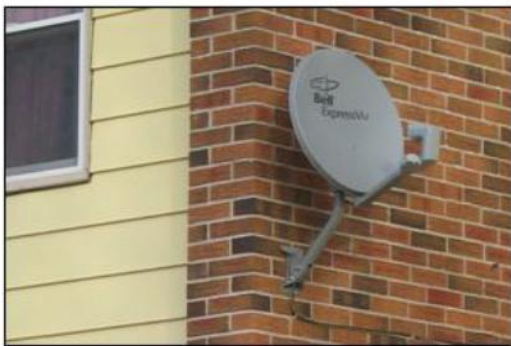
Fastened to Brick Wall Outside Unit
