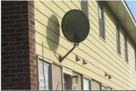
Fastened to Siding
